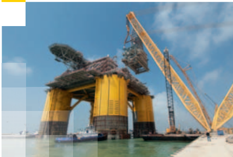
Construction of the Olympus platform for the Mars B development in the USA.
