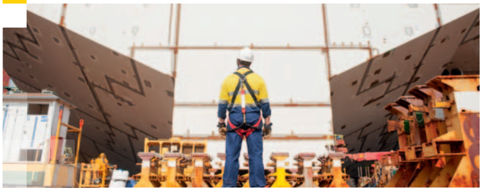
The hull of our Prelude floating liquefied natural gas facility under construction in the Geoje shipyard, South Korea.
