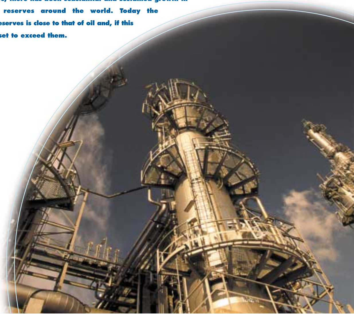
Distillation columns of the SMDS plant in Malaysia
