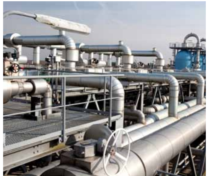
Gas Storage Norg, Netherlands, 2010
