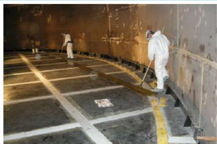
Internal Floating Covers are the largest (in scale) environment improvements delivered at the refinery.
