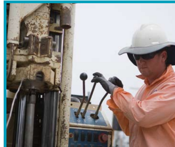
In an Australian first, innovative drilling tools and techniques are being used at the refinery.
